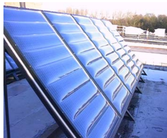
Filsol flat plate system on Wedgewood Visitor Centre (photo courtesy of John Blower), serving washrooms
