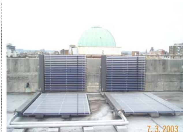
Viessmann evacuated tube system, London Borough Of Camden (photo courtesy of LB Camden), serving washrooms for office accommodation, library and health centre.
